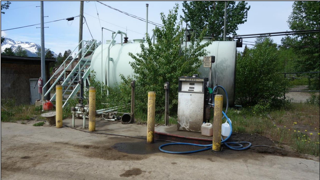
Photograph 5: Diesel AST for powerhouse/generators and Enterprise Works Yard fuel pump, located northeast of the Band Office, looking southwest
