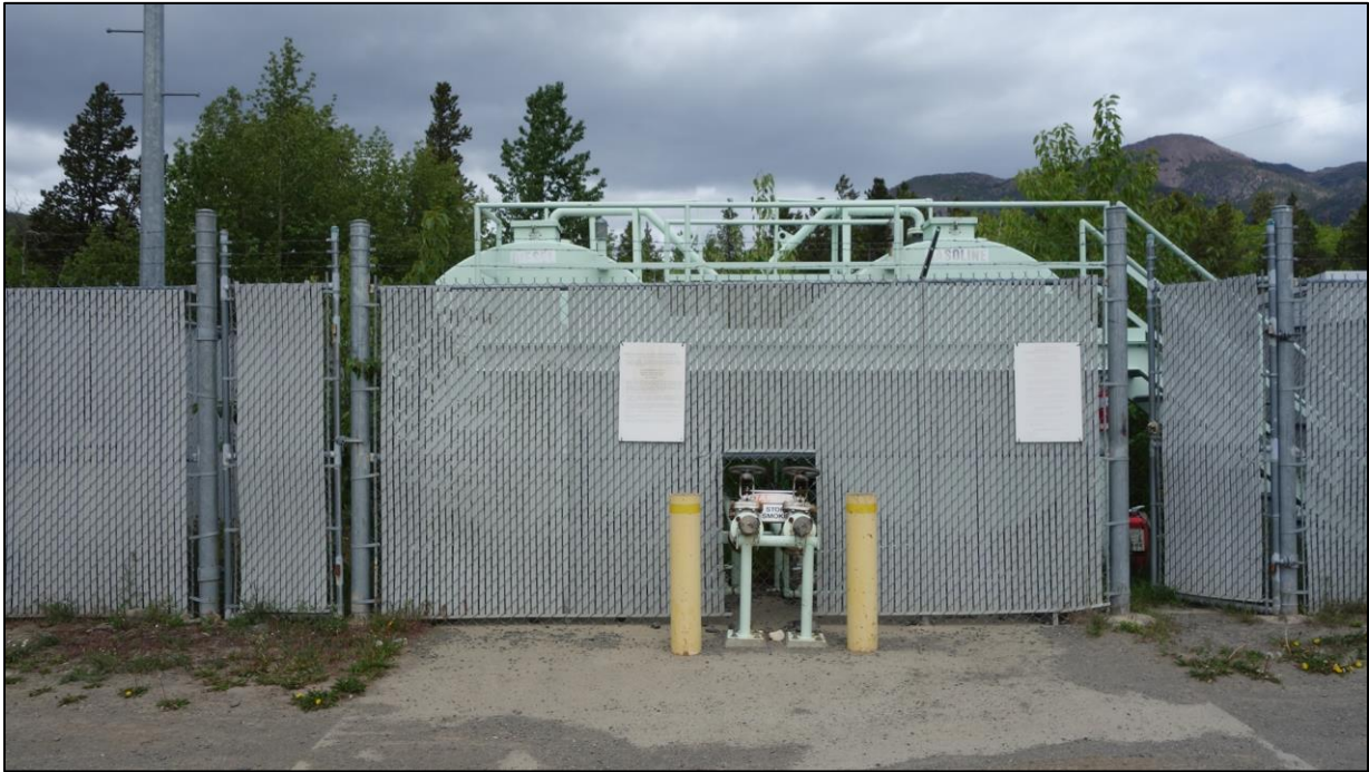
Photograph 11: Enterprise gas station ASTs looking north
